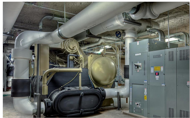
Inside mechanical room
